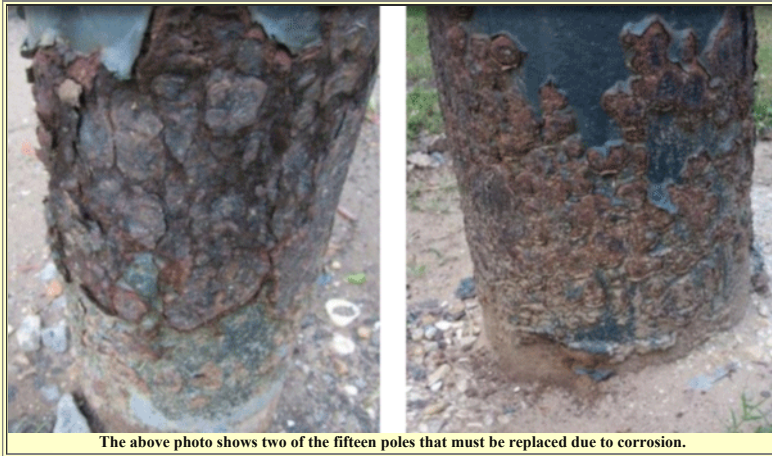
The above photo shows two of the fifteen poles that must be replaced due to corrosion.
